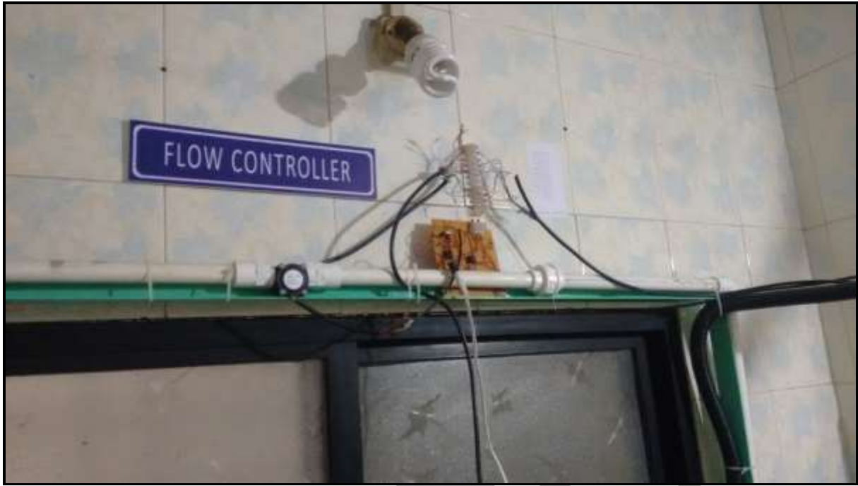
Flow Controller used in PLC
