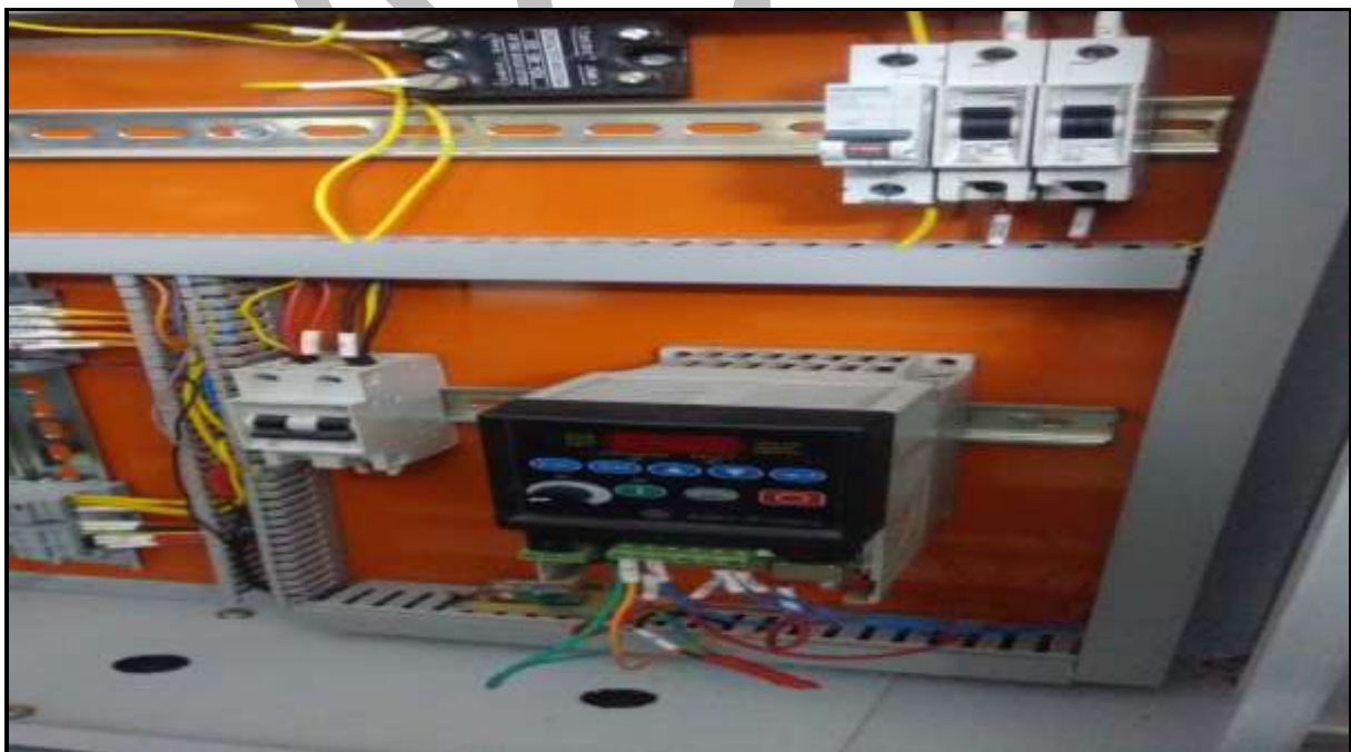
Variable Frequency Drive (VFD) USED IN PLC
