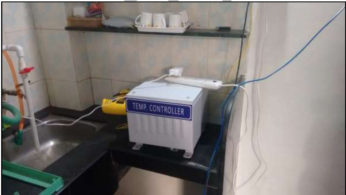
Temperature Control by PLC
